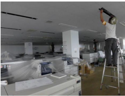
Conversion to LED lighting
