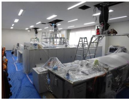
Introduction of energy-saving air-conditioning equipment
