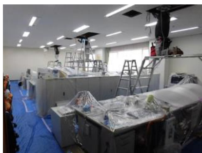
Introduction of energy-saving air-conditioning equipment
